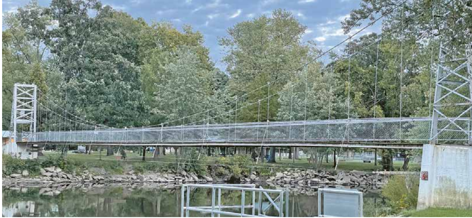
Over the next month or so, Southern Road and Bridge will be working on repairs to the Memorial Swinging Bridge. The bridge will be closed for the duration of the project - from the morning of Sept. 27 to approximately Oct. 31. A $239,000 bid from Southern Road and Bridge was approved in July for the work on the bridge, which includes new decking, painting, welding and other general repairs. The Winamac parks board will put $43,000 towards the repairs and the town of Winamac will cover $86,000. A $110,000 anonymous donation is expected. Shown above, workers will be able to walk both on and underneath the bridge to make the necessary repairs.
